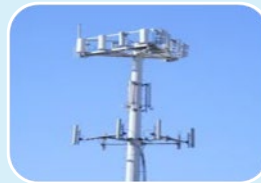
Cell towers/ antennas
